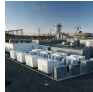
SOLAR & STORAGE SOLUTIONS
